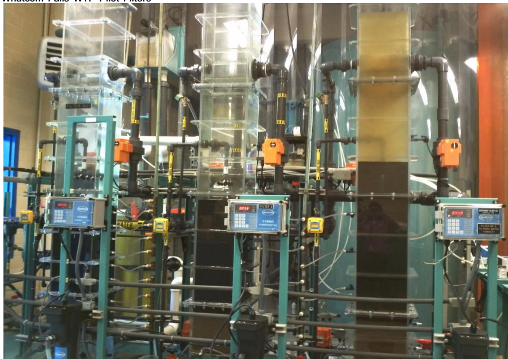
FIGURE 2-4 Whatcom Falls WTP Pilot Filters
