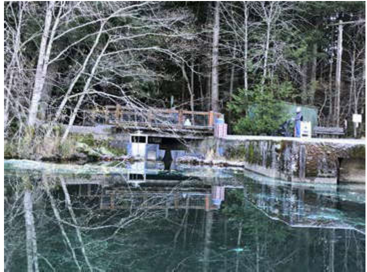
Figure 2-10. Lake Padden outlet structure
