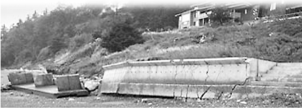
Figure 6. Failed bulkheads and large slide on Whidbey Island (Washington Department of Ecology http://www.ecy.wa.gov/programs/sea/pugetsound/building/bulkhead.html )
