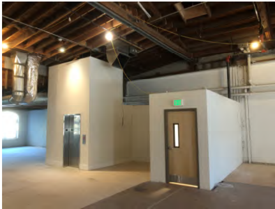
Second Floor Elevator
