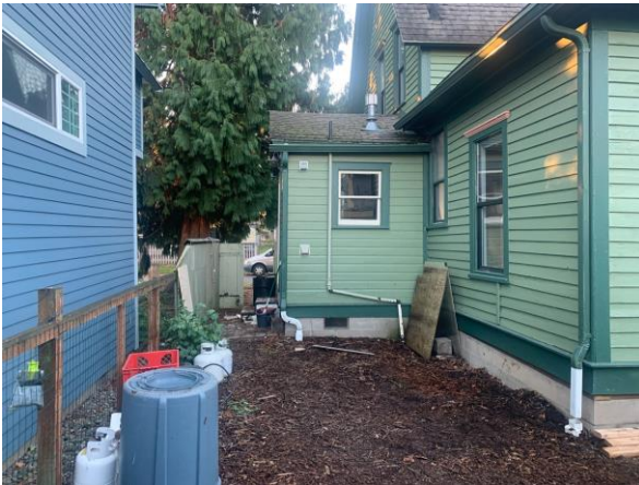
Before - different siding style on laundry room
