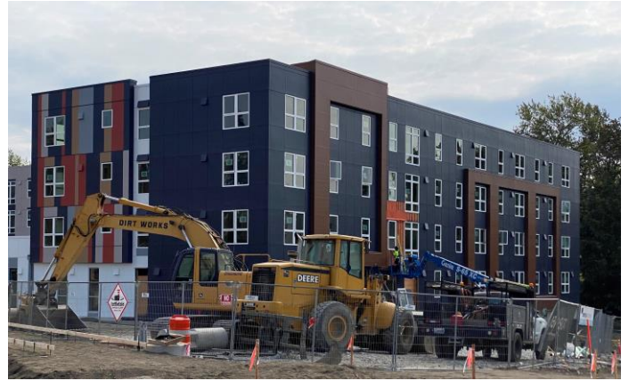
L: BHA Samish Commons under development R: MHNW Trailview Housing under development Photos by Samya Lutz
