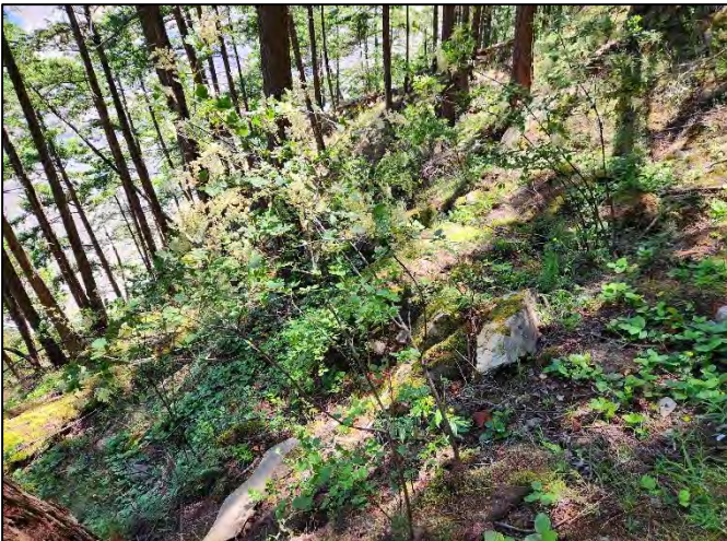
Photo 11: Slope face below fractured outcrop. Note rock fall debris in foreground.
