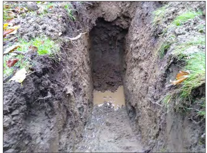
Photo 4: TP2 Caving on South Pit-Wall
