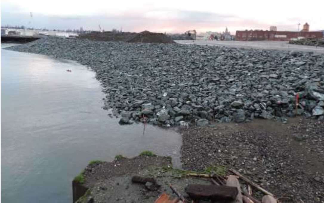
Photo 13. Study site 6 after a revetment was constructed along this shoreline. This work was completed to protect the redevelopment of the Waterfront District.
