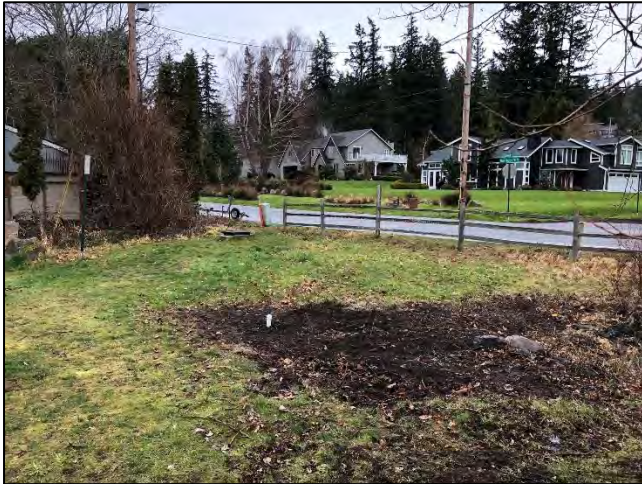
Photo 7: Boring location B5 at the north end of the site with well casing installed. (2-8-22)
