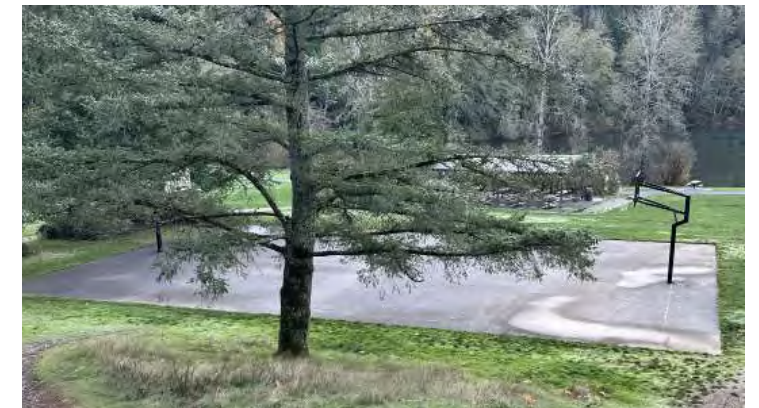
Basketball court- striping is very faded and concrete has numerous cracks- condition rating 4.
