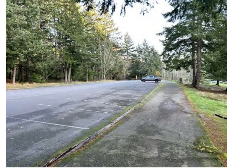
Pavement and sidewalk in poor condition rating 4.
