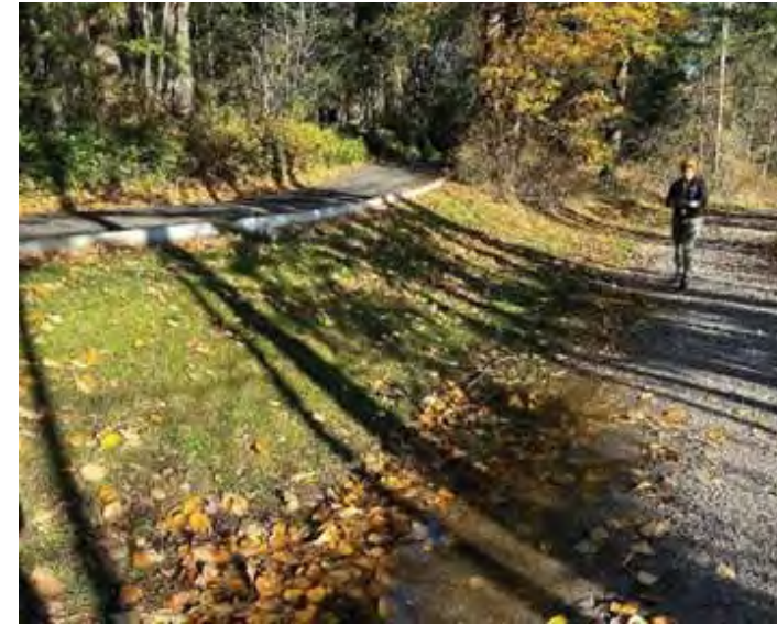
Figure 27. Main loop trail segment with drainage issues in Zone 4.
