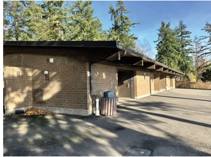
Bath house- condition rating 3.
