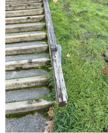
Wood handrails in poor repair on parking lot stairs- condition rating 4.
