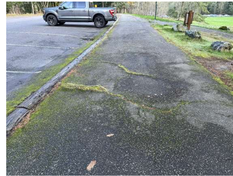
Wood edging presents barrier to movement between parking and sidewalk.
