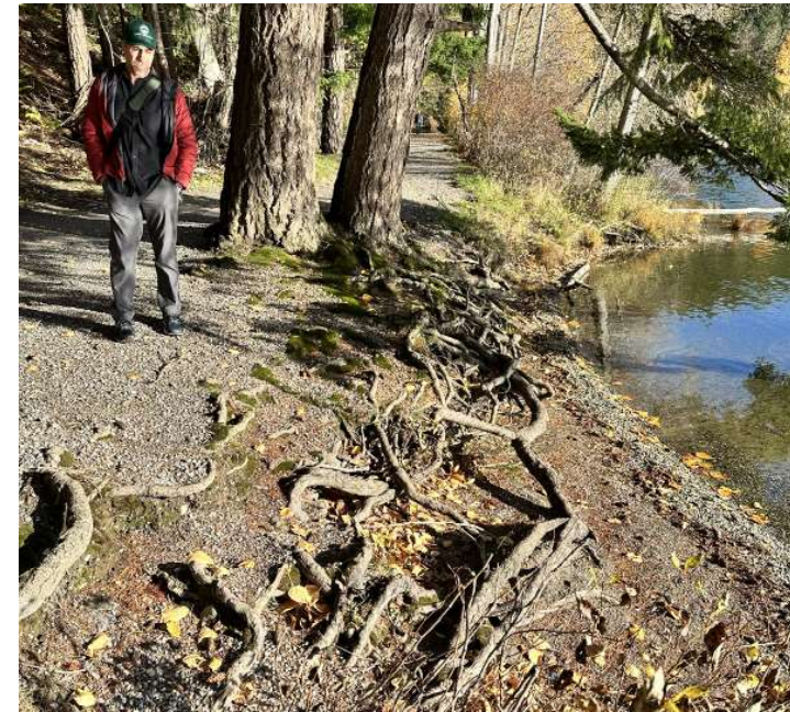
Bank erosion on east shoreline.
