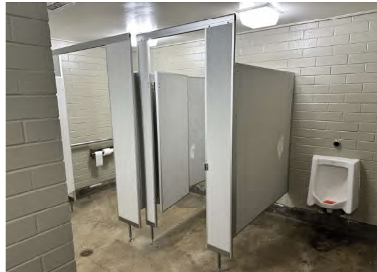
Bath house interior- condition rating 3.
