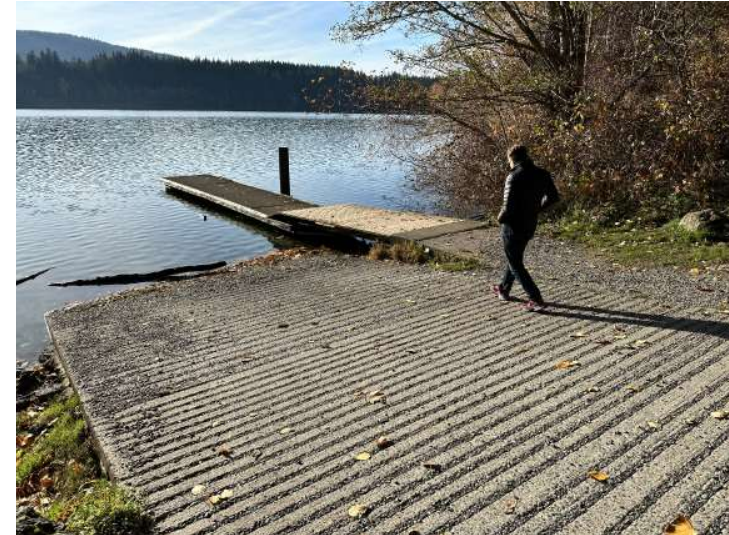
Boat launch ramp and dock- condition rating 3.
