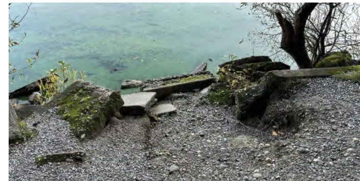
Shoreline edge erosion and historic debris- condition rating 4.
