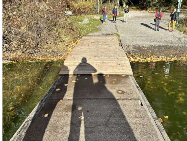
Boat launch ramp and dock- transition is not ADA accessible. Dock lacks toe kick rails.
