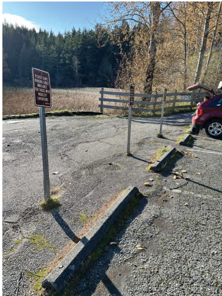
Fishing area accessible parking- condition rating 5.
