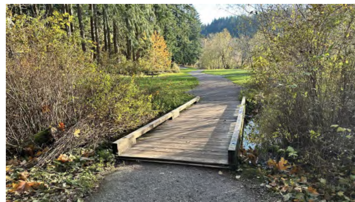
Pedestrian bridge transition is not ADA compliant.
