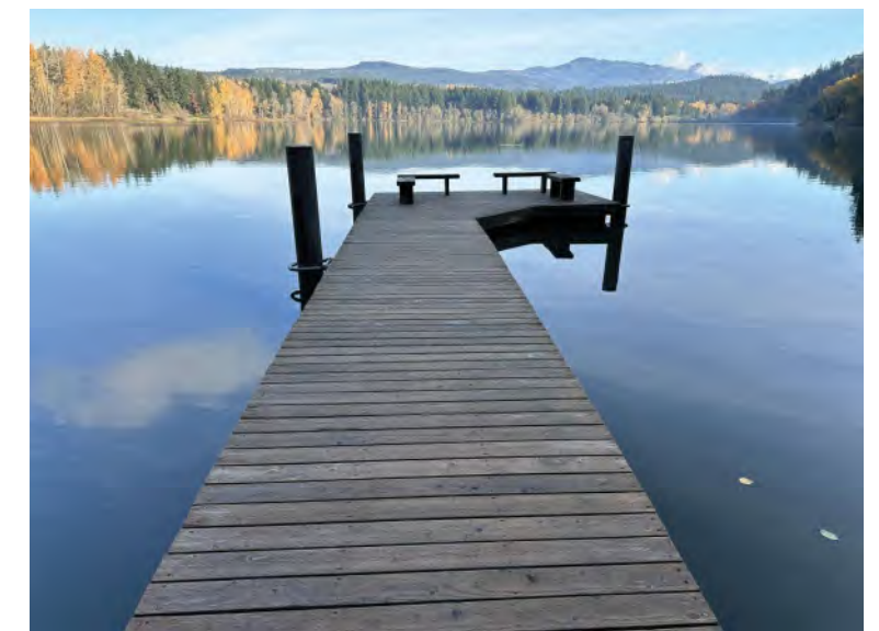
Fishing dock- condition rating 4.
