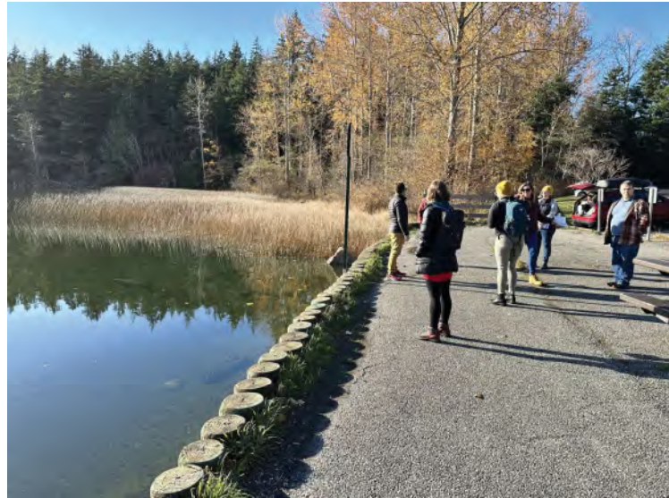
Fishing area bulkhead- condition rating 4.
