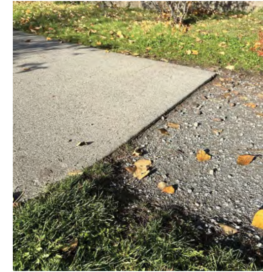
Transition between improved trail and concrete pathways not-ADA compliant.
