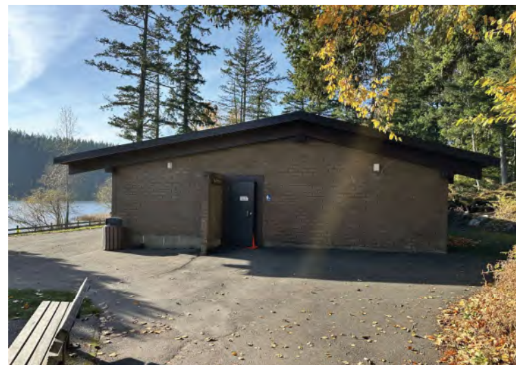
Bath house- condition rating 3.
