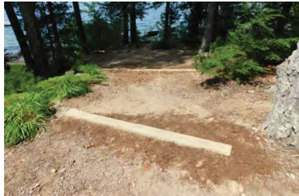
Figure 38: Trail waterbars to control path erosion
