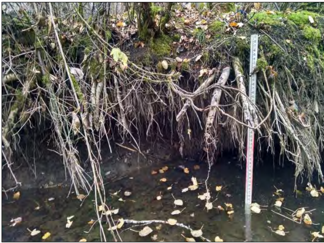
Photo 23: Severe undercut bank behind Hospital.
