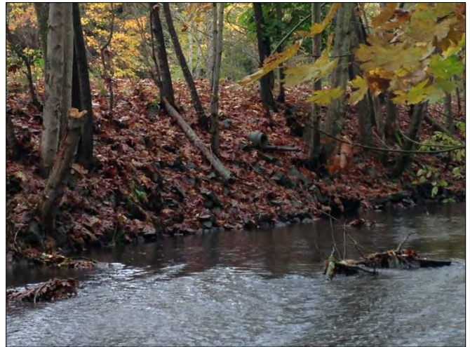
Photo 4: Relict bank armoring.
