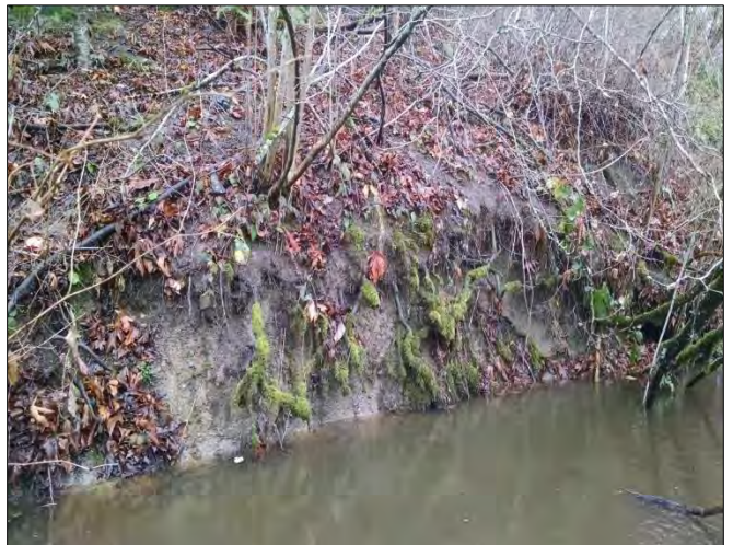
Photo 16: Bank erosion in reach B-5.
