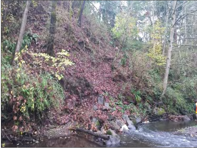
Photo 1: Active Erosion site, partially armored.
