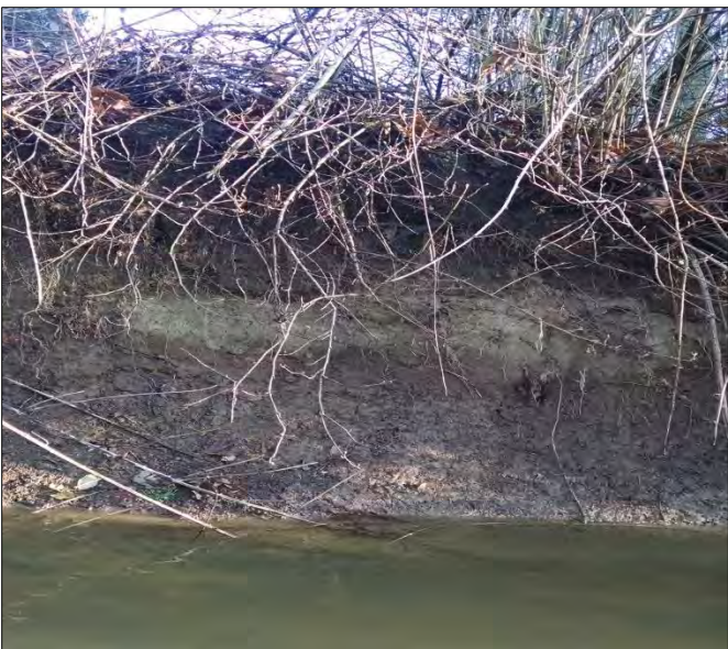
Photo 25: Active erosion in D-6.
