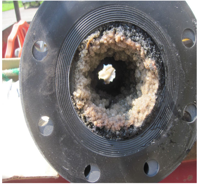
Figure 2-1. Nuisance Struvite Formation within Piping
