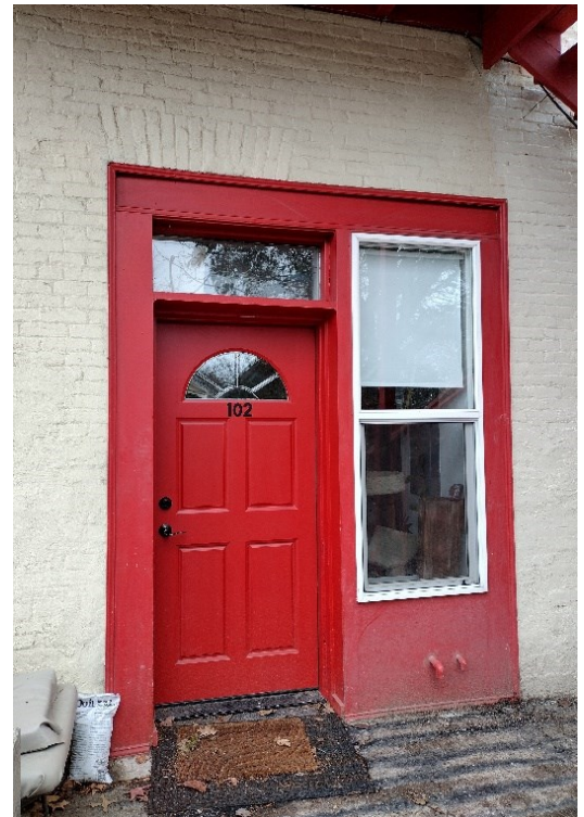
Figure 19. Note the vertical brickwork over the entry door to Apartment 102 under the stairway on the southwestern face, revealing the expansion of the opening to include a window next to the door.
