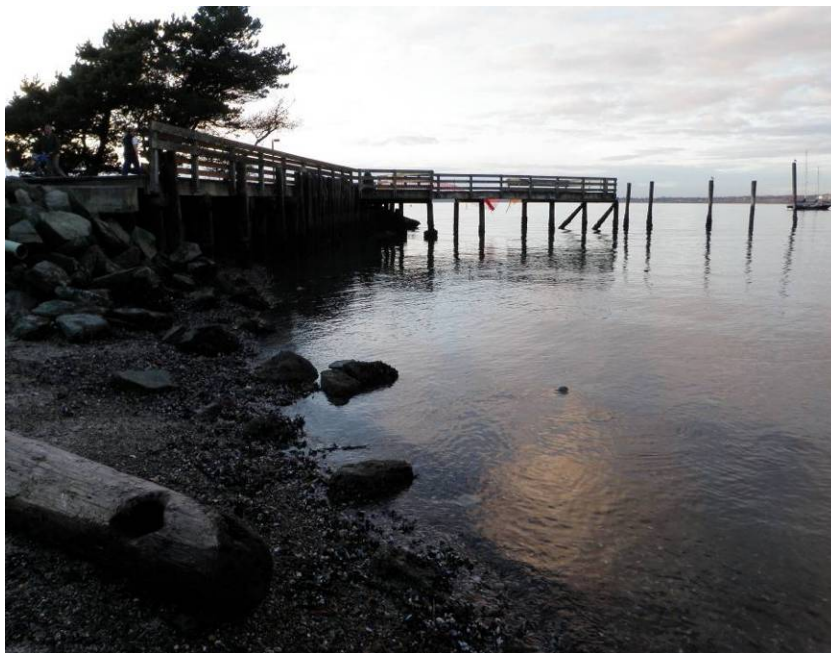
Photo 1 – Profile view of the existing pier at Boulevard Park from the adjacent pocket beach located at the northeast corner of Boulevard Park (facing west)
