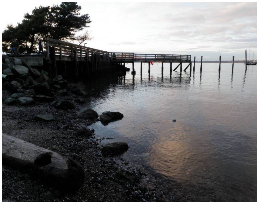
Photo 1 – Profile view of the existing pier at Boulevard Park from the adjacent pocket beach located at the northeast corner of Boulevard Park (facing west)
