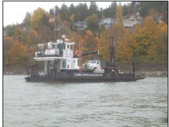
Six geotechnical borings were completed from an anchored barge using a subcontracted truck-mounted drill rig.
