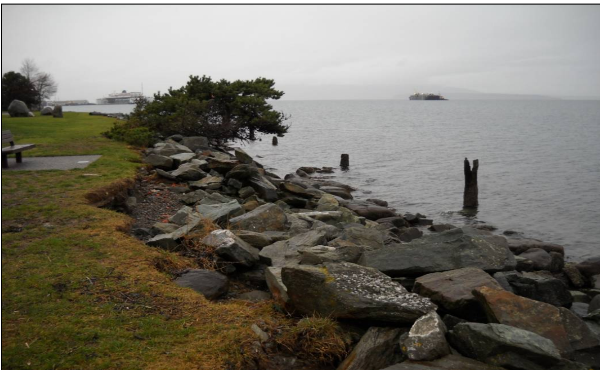
Old pilings southwest of the existing dock at the northern end of Boulevard Park, Bellingham, Washington. View is to the southwest.
