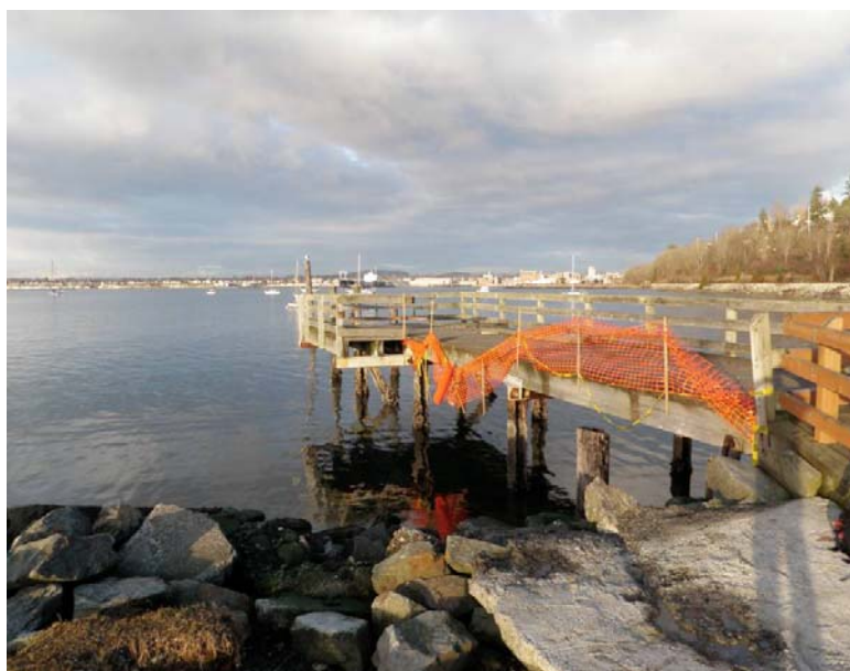
Photo 1 – View from Boulevard Park of the existing pier where the southern end of the overwater pedestrian walkway will land (facing north)
