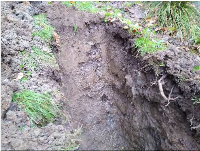
Photo 3: TP2 Seepage from North Pit-Wall
