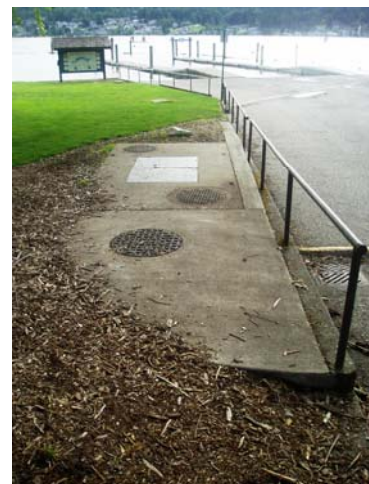
Media filter stormwater treatment facility
