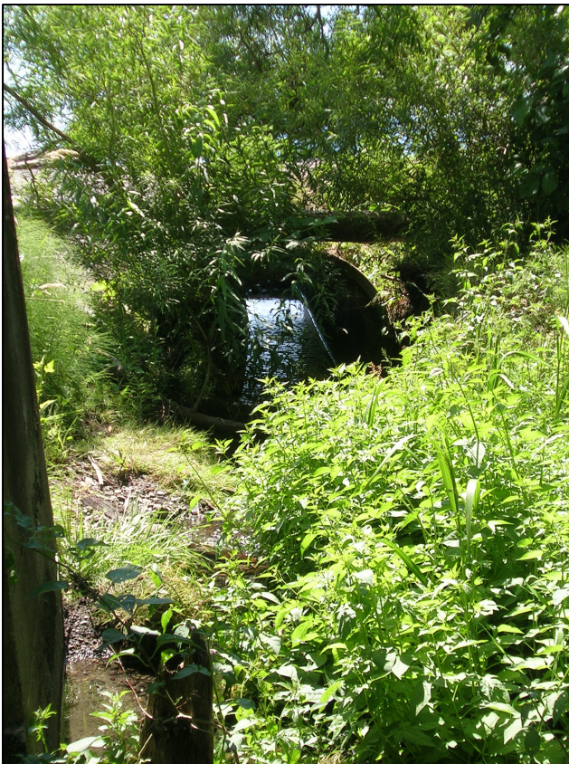
Little Squalicum Creek culvert under trail to Little Squalicum Beach as seen facing south forest (June 2009).
