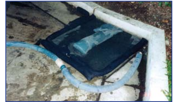
A storm drain cover with vacuum hose.
