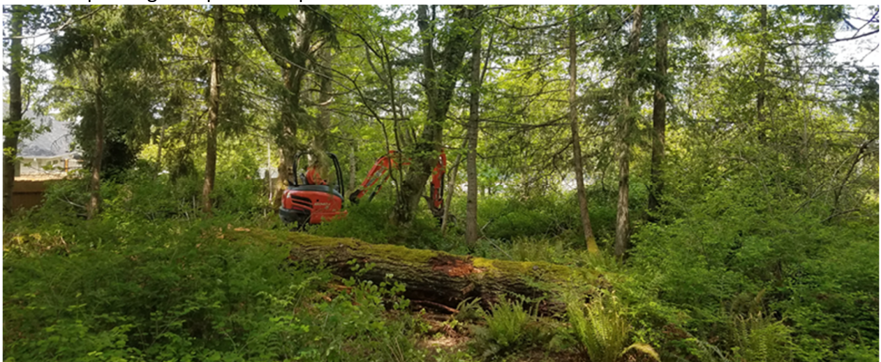
Image 1 – Typical surface conditions of site interior. View facing north with test pit TP-9 in progress.
