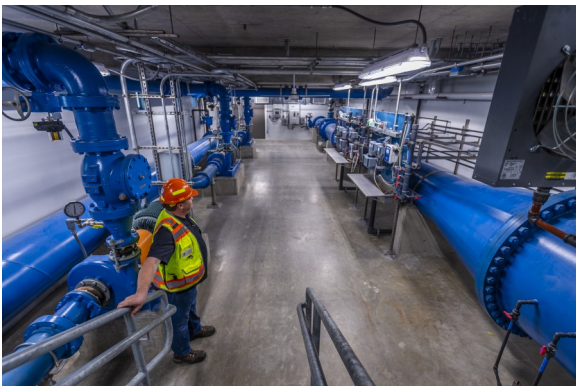
Operator below the filter gallery at the Water Treatment Plant
