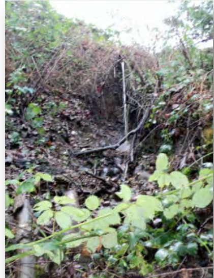
Photo 9. Failing outfall below (north) Old Lakeway Drive.
